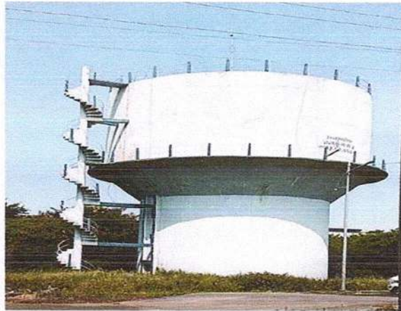
Fig. Elevated Storage Tank Of 13,50,000 Lit Capacity Each.
