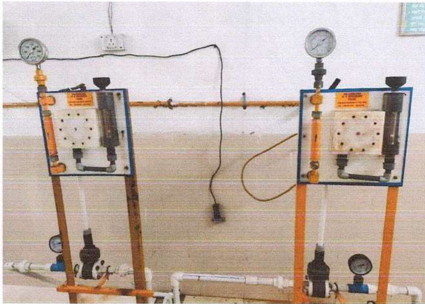
Fig. Chlorination Process Unit.
